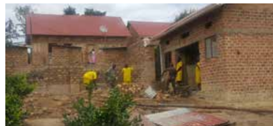
▲ Top: Renovated building at Mbale Remand Home Middle: Inmates laying bricks at Orom Tikao Prison Farm in Kitgum district Bottom: Inmates constructing a hall at Rakai Prison
