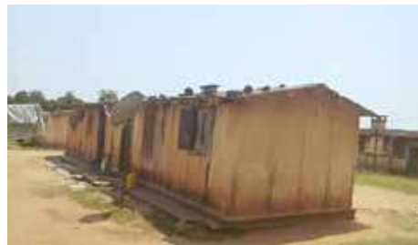
◀ Dilapidated police accommodation at Kitgum Police Station
