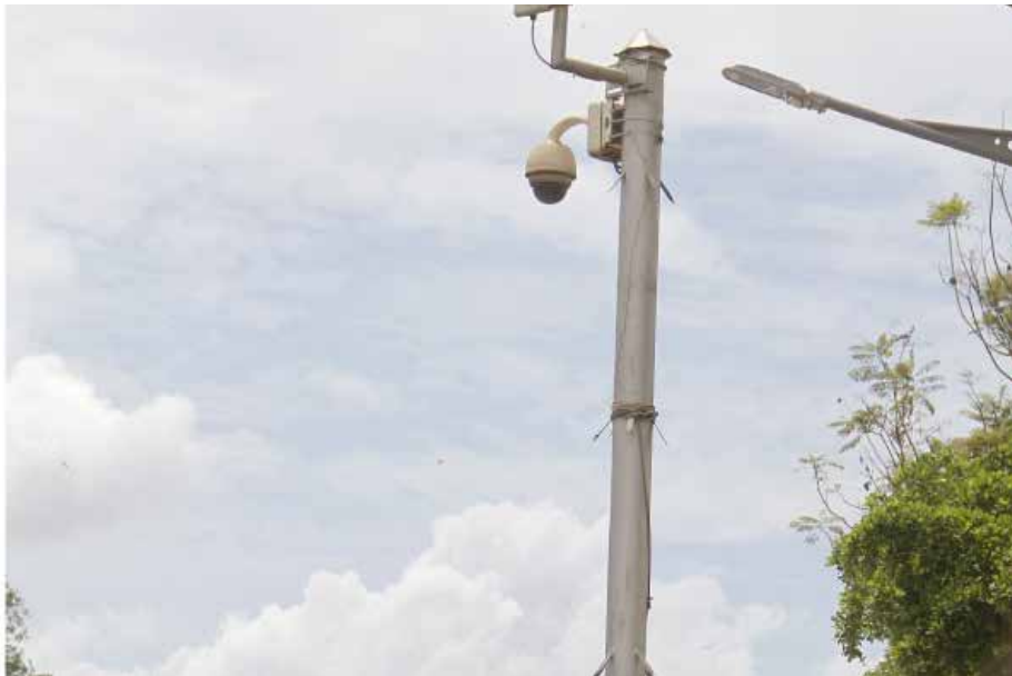
◀ Street camera at Jinja Road traffic lights. Similar cameras have been installed in and around Kamapla and Wakiso to reduce crime in the city
