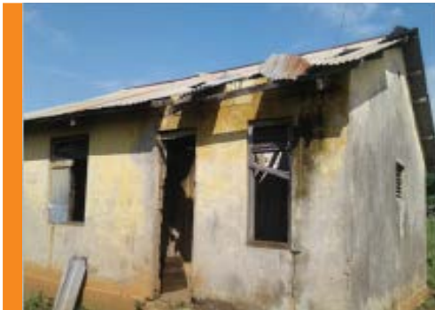
Dilapidated police office at Agwata Police station
