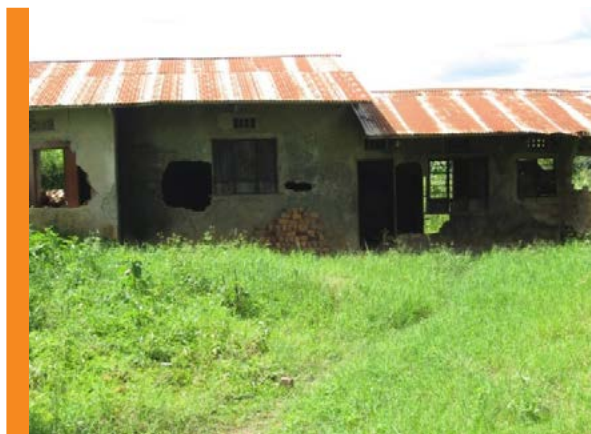
A family house in Muduuma sub-county, Mpigi district that was allegedly destroyed during a land dispute
