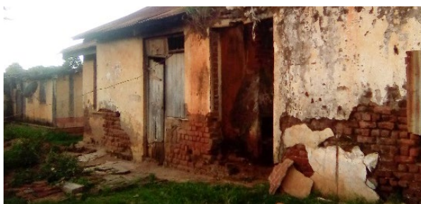
Old and dilapidated staff accommodation at Kitgum Central Police Station
