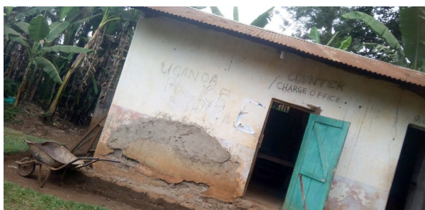
Dilapidated structure at Bulucheke Police Post in Bulambuli District
