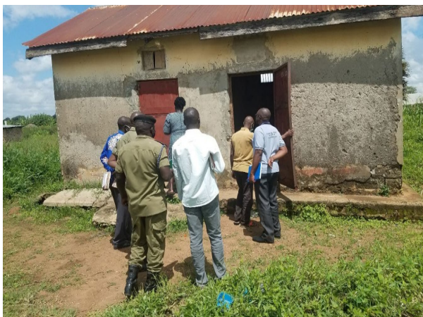
UHRC officials inspecting dilapidated cells at Kochgoma Police Station in Nwoya District
